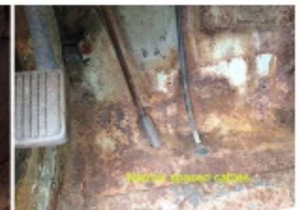
Wide spaced cables
